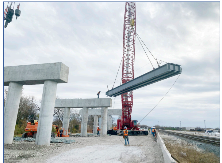
Construction team placing structural steel for the Forest Hill Flyover (P3) Project.
